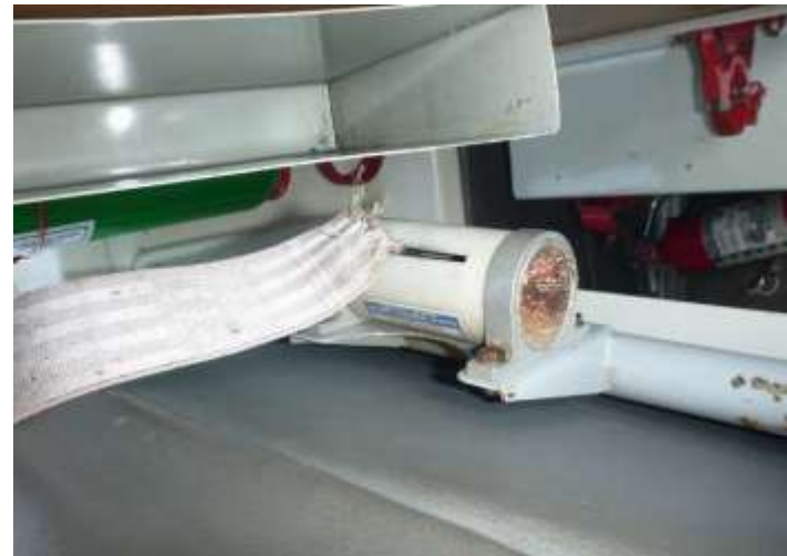
Failure of top strap
